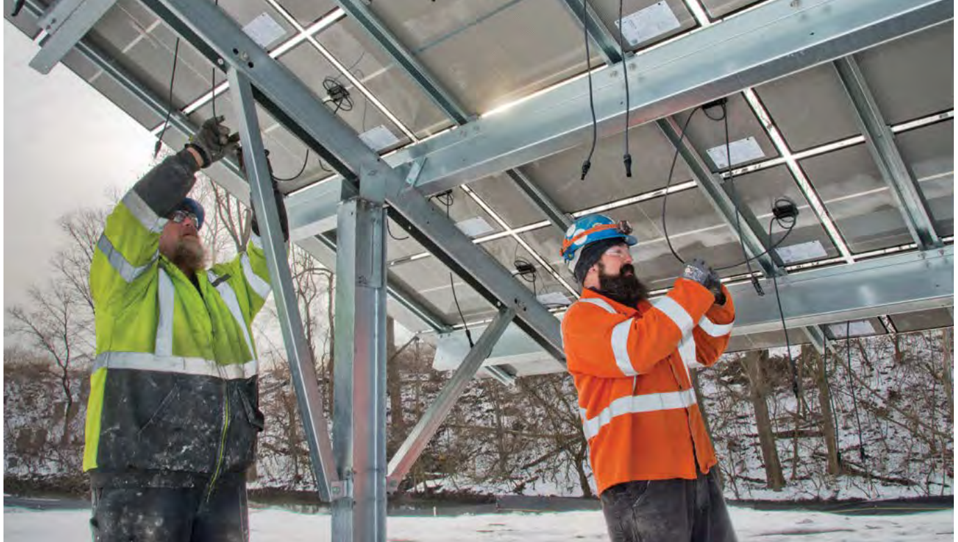
GEM, Inc. employees Joe Rybka and Ryan Schmitt install solar panels on the Overland site.
